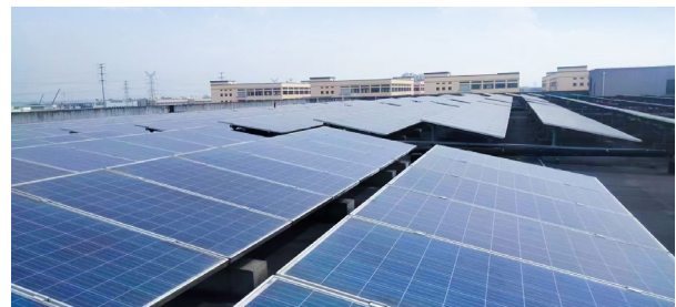
The photovoltaic power generation equipment installed in Joyoung factories and offices.
