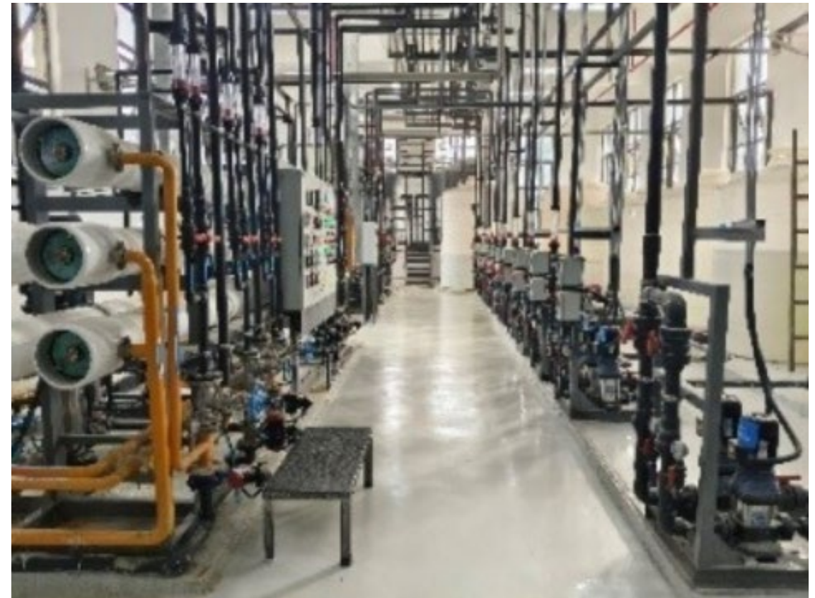
Wastewater treatment station
