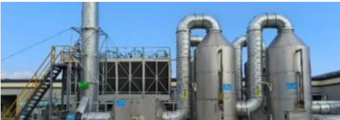
Air emission treatment facilities
