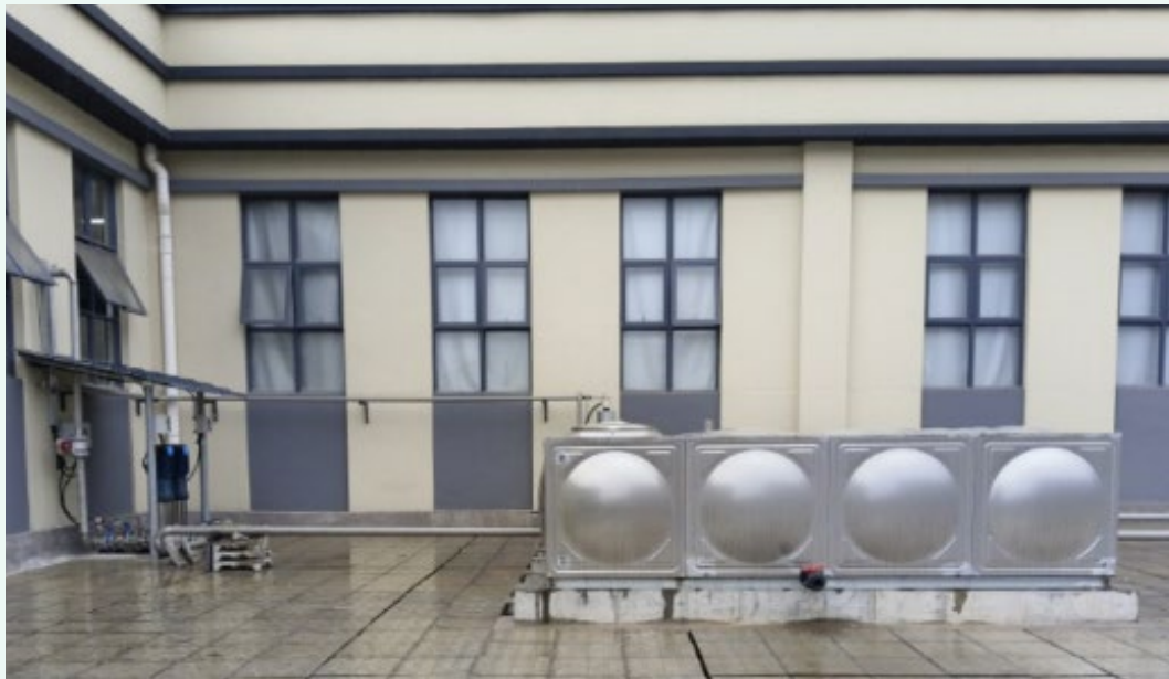
Huizhou Highpower Production Waste Water Recovery Project
