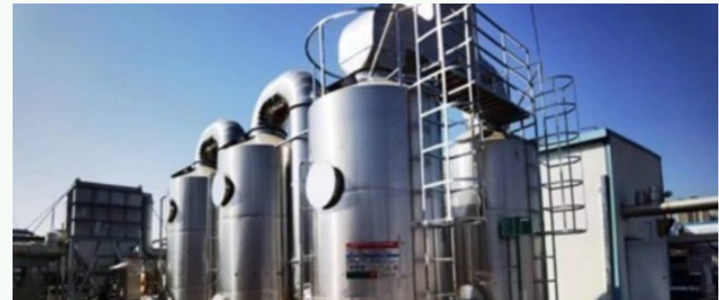
Reconstruction of NMP air emission treatment equipment
