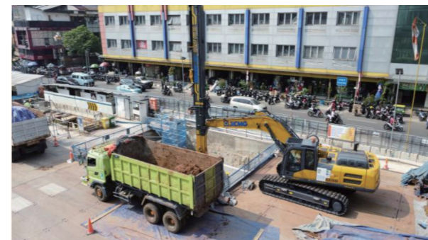
Jakarta MRT Project Several XCMG XEG2600 telescopic excavators were contributing to the construction of the second phase of the Jakarta MRT North–South Line project. Serving as pioneers in this infrastructure endeavor, they were tasked with the critical role of initial earth excavation.
