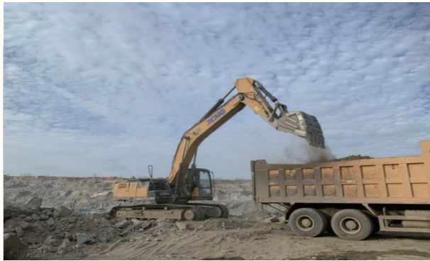
Swak Dam Project in Kenya 13 XCMG XS263S road rollers were supporting the construction of the Swak Dam in Kenya. The dam's civil engineering in which XCMG Machinery played a role covers a stretch of about 1.5 km, with a total embankment volume of approximately 12 million cubic meters.
