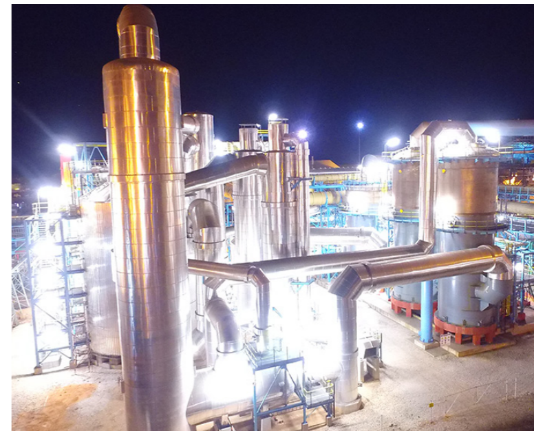
Tsumeb Smelter 烟气制酸设施
