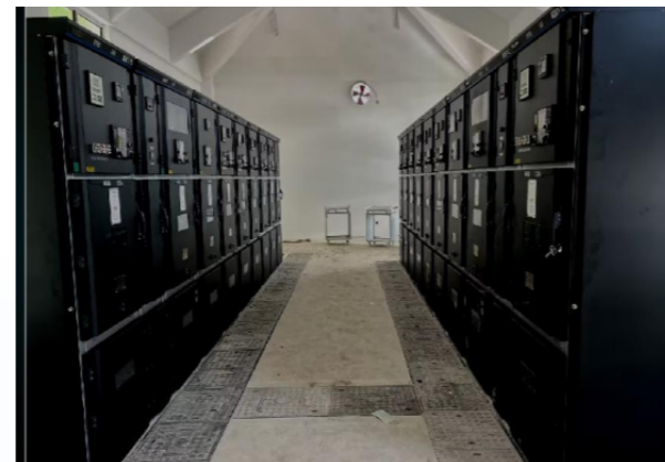
Intelligent distribution room of Hubei University
