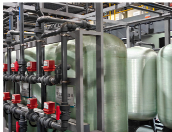
Wastewater treatment facilities
