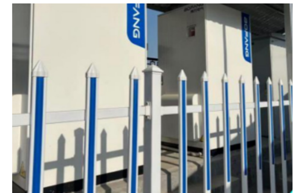
522kWh energy storage station
