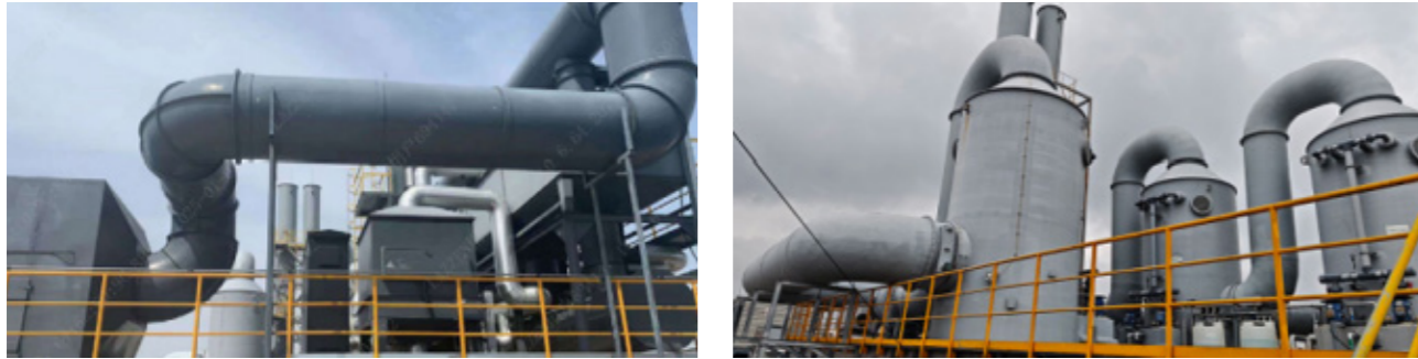
Waste gas treatment facilities
