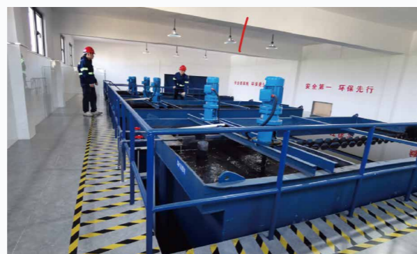
Reclaimed water reuse facilities
