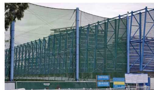
A new steel windproof and dust suppression mesh has been constructed at Shihushan Terminal. By employing aerodynamic principles, the wind and dust suppression wall is designed to create upward and downward airflow disturbances on the inner side of the wall, effectively preventing dust from spreading beyond the site.
