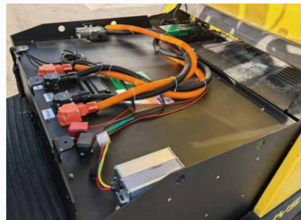
Upgraded Lithium Battery Pack
