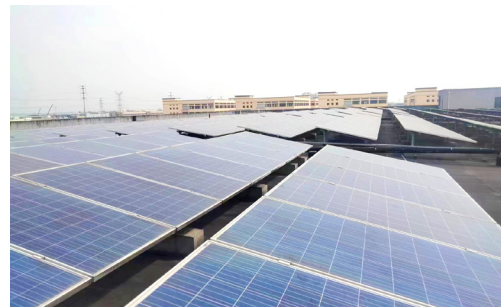
Rooftop PV Power Generation Equipment at the Hangzhou Campus
